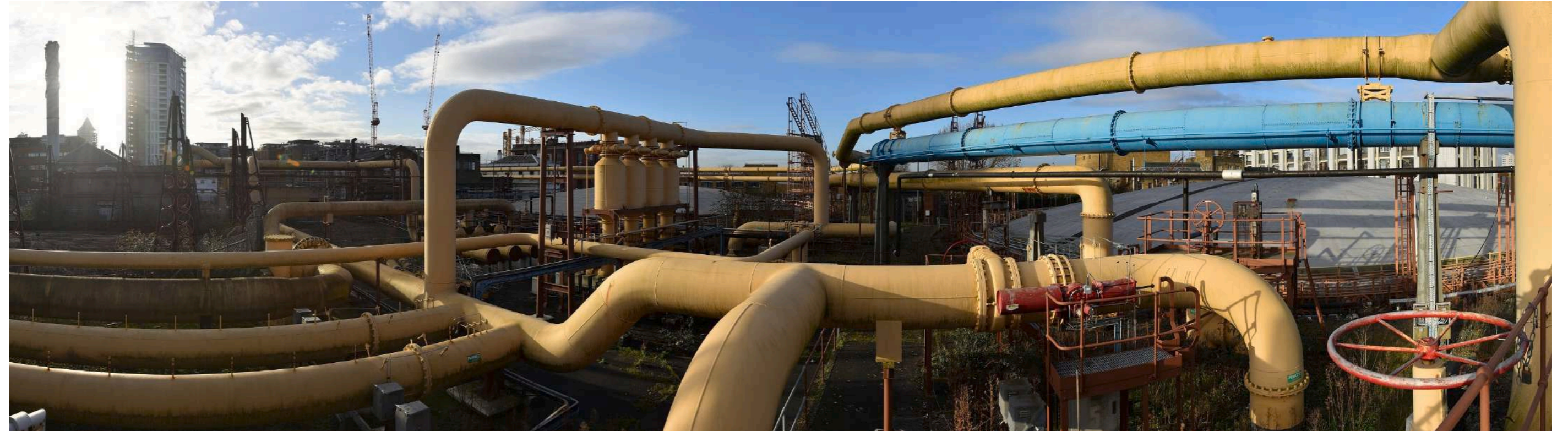
Redundant Gas Equipment, Fulham Gasworks
